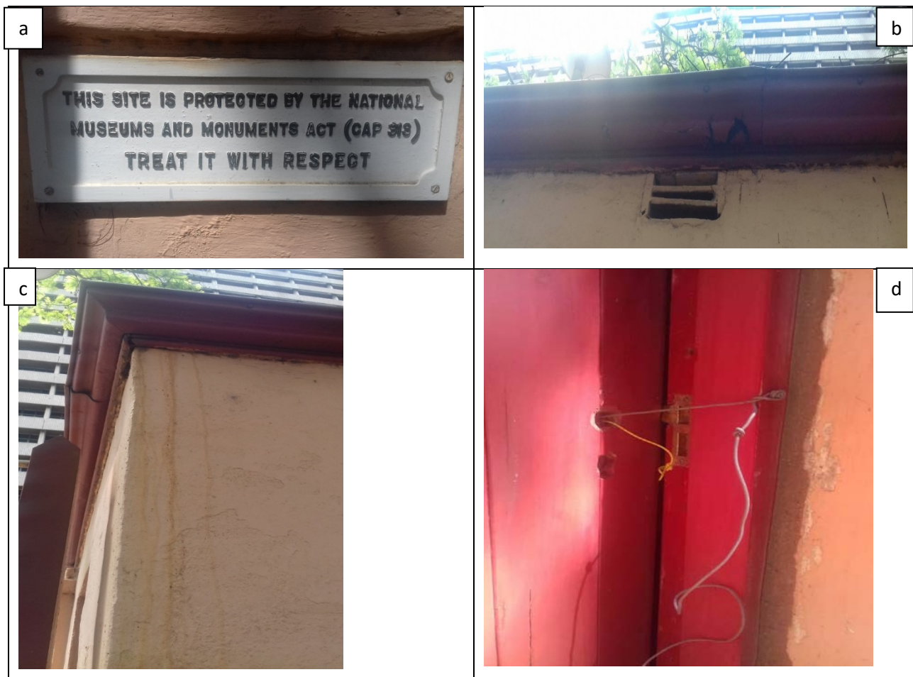
Figure 12: shows state of maintenance of Mother Patricks mortuary. a: an outdated signage of a national monument, b: shows leaking gutters, c: shows leaking roofs, d: shows an unfixed door. Photos by BM.
